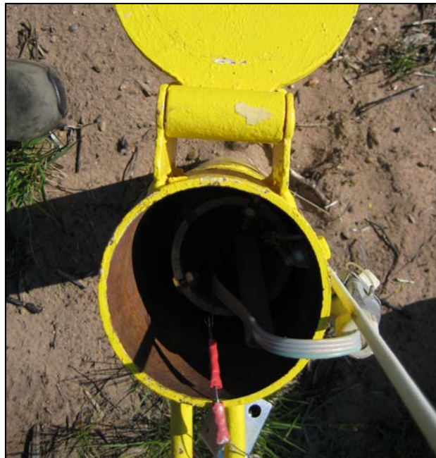
Piezometer with a level troll located at QAL008A
